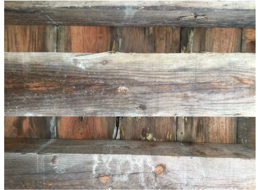
Indication of rot on subdeck - cored and fair condition
