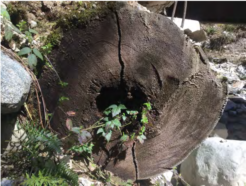
Vertical crack in crib log on right bank
